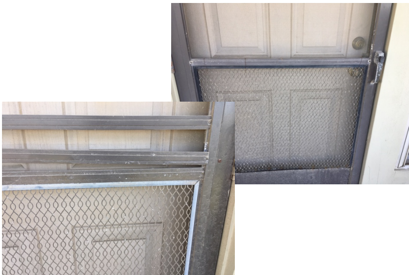
Examples of Screen Doors Needing Replacing
